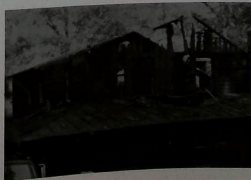
Buffalo Lodge after the fire in May, 1973. Though major damage was done to the east portion, renovation of the building will be completed in time for use by summer camp, 1974.
