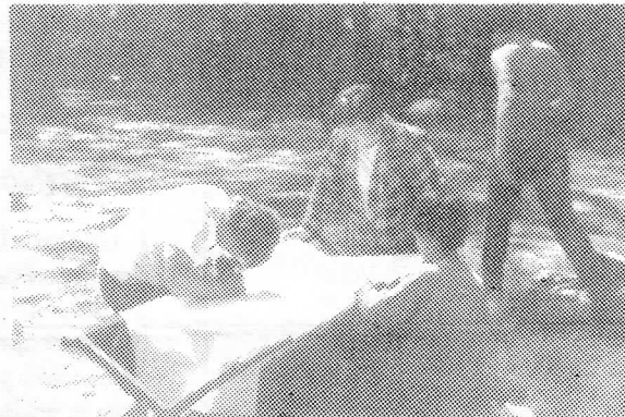
Right: Whether its fixing cots & tent platforms, painting, trail maintenance, carpentry, wiring or plumbing, the Lodge does its best to help maintain our Council Camps.
